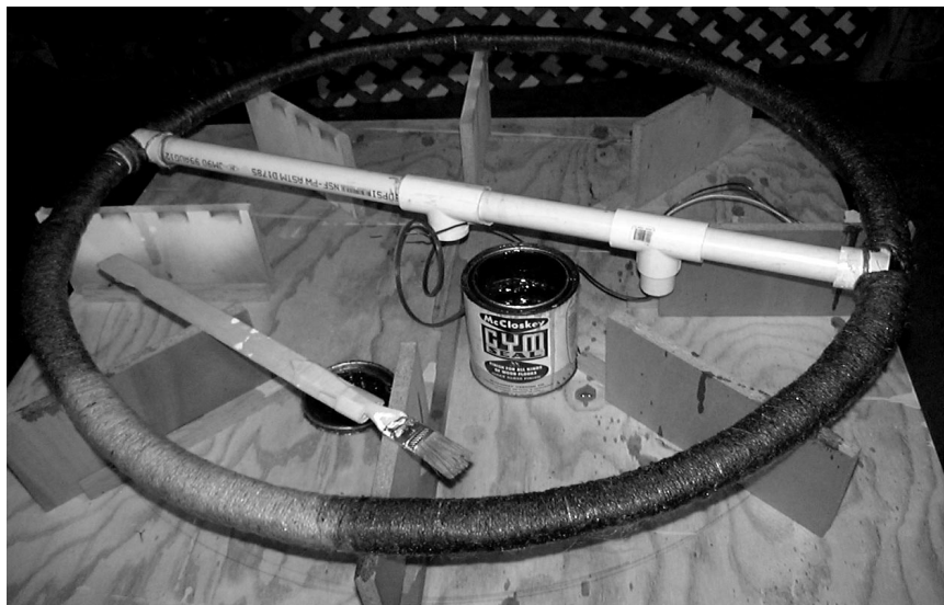
Figure 39-15 Loop construction almost done, first coat of varnish almost complete. At lower left can be seen the light-brown jute wrapping. Jute turns darker with varnish. A can of McCloskey Gym Seal petroleum-based varnish is in the center. Final assembly wound up with three coats of varnish, allowing a week of drying between each coat. Final coating exhausted a quart can of varnish.
