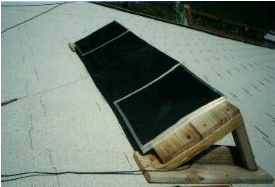
Solar panel on the roof
